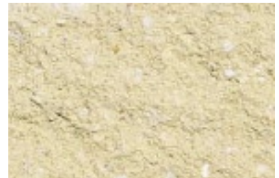
Rough surface finish on wall to discourage graffiti and vandalism
